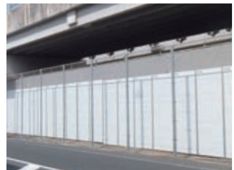
Temporary Soundproof Panel
