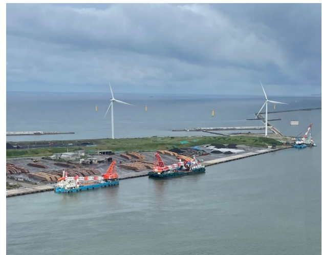
Offshore wind power generation business
